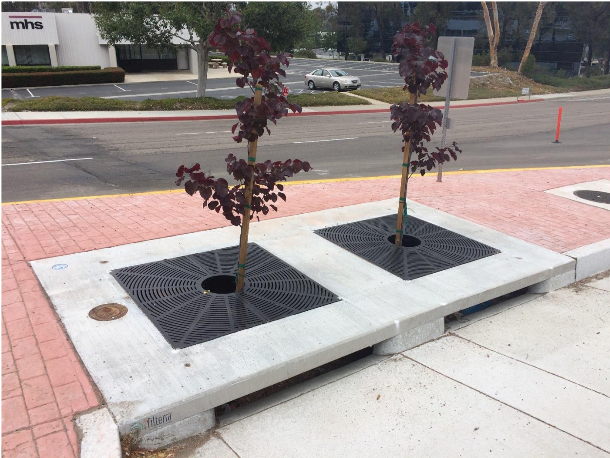
Figure 2. Tree box incorporated into a storm drain inlet in San Diego, CA
