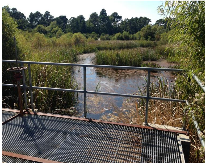
Figure 2. Constructed wetland inlet.
