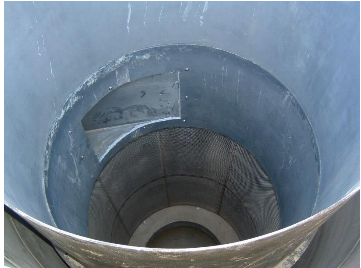
Figure 1. Looking down a hydrodynamic separator from the top where stormwater tangentially enters the unit.
