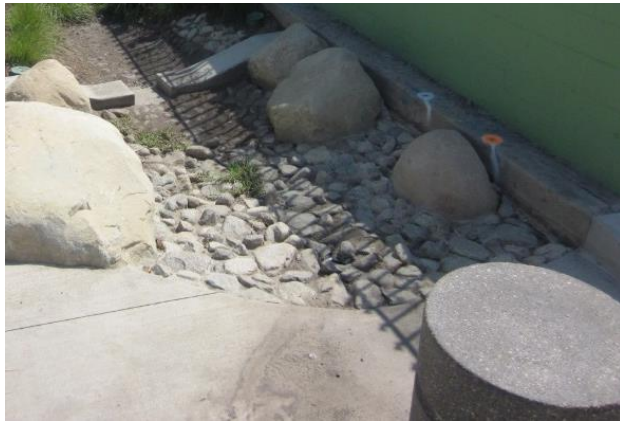
Figure 3. Example of a forebay as pretreatment
