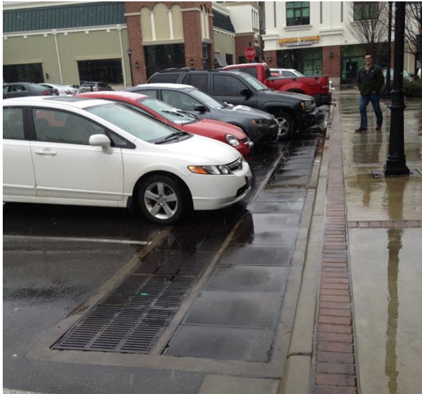
Figure 1. Example subsurface inlet in parking lot.
