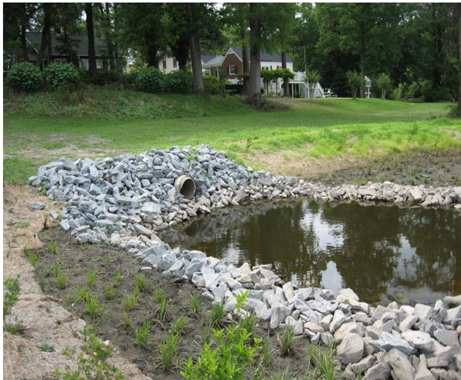
Figure 1. Example forebay. Also note other components of the pond: earthen berm and native vegetation
