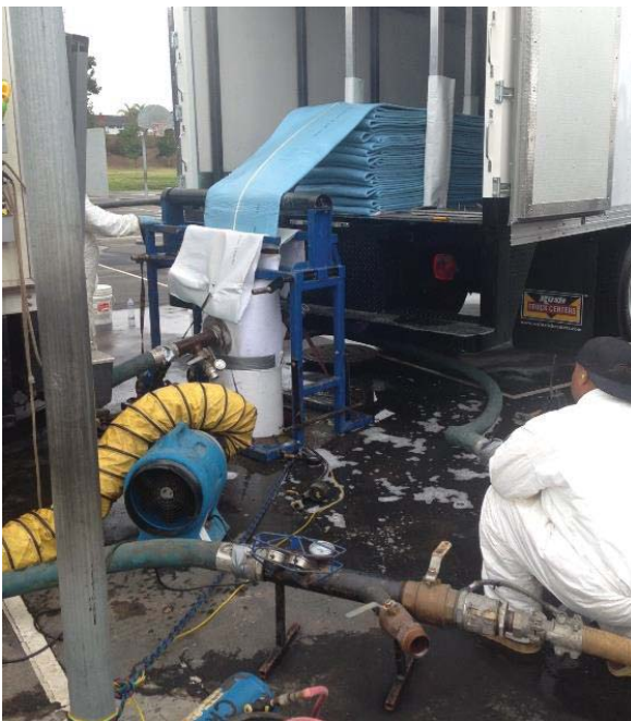
Installing Cured-In-Place-Pipe (CIPP) slip lining to rehabilitate the City's pipelines and protect against leakages and water quality contamination.
