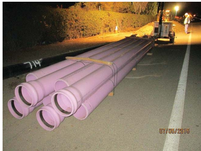
Installation of recycled water pipelines constructed as part of the Recycled Water Conversion and Pipelines Project
