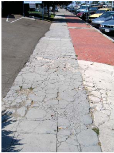
3A) Some of Oceanside's sidewalks are in disrepair and represent both trip hazards as well as accessibility issues. Shared cost programs to repair and replace damaged sidewalks do exist. Photo credit: Mike Singleton
