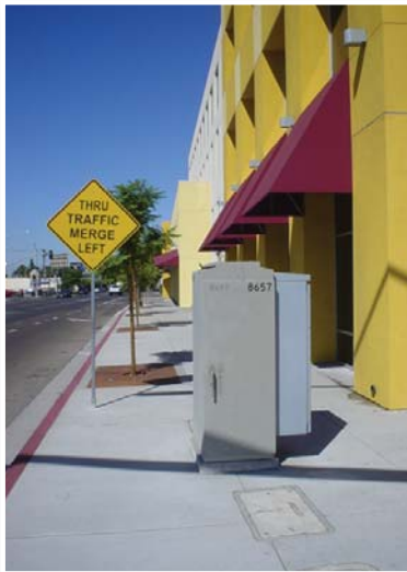
4A) Even though this project provided a wide walkway to start with, some equipment has been placed outside of the furnishing zone and in the throughway zone. Photo credit: Andy Hamilton
