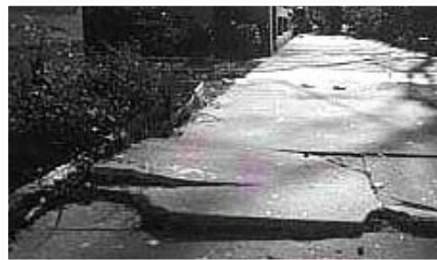
7A) Repair, slice or patch lifts on walk surfaces and/or reset ground level utility boxes to be flush. Photo credit: Mike Singleton
