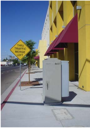
4A) Even though this project provided a wide walkway to start with, some equipment has been placed outside of the furnishings zone and in the throughway zone. Photo credit: Andy Hamilton
