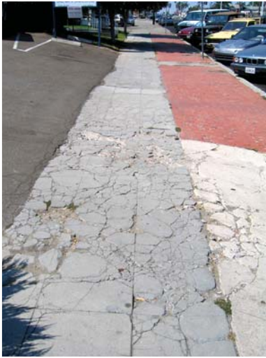
3A) Some of Oceanside's sidewalks are in disrepair and represent both trip hazards as well as accessibility issues. Shared cost programs to repair and replace damaged sidewalks do exist. Photo credit: Mike Singleton
